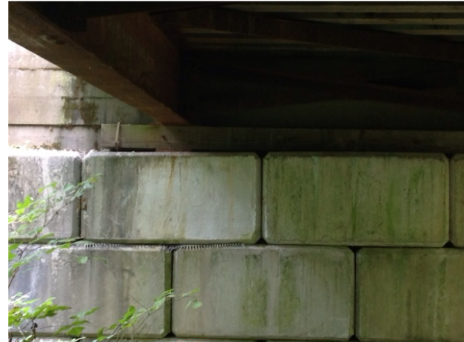
right downstream bearing shimmed
